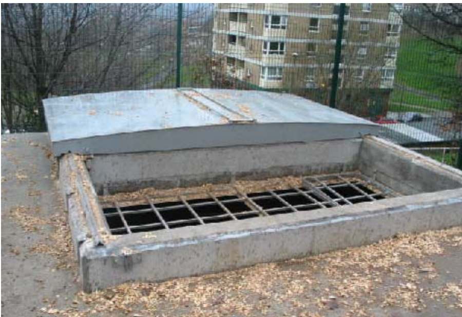
Manual push-back bunker lid awaiting a fuel delivery
